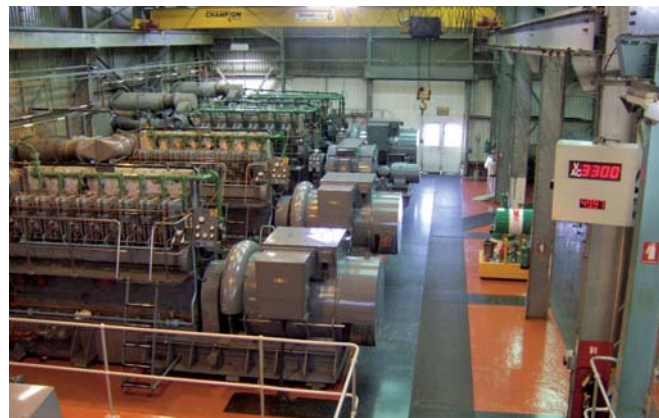
Generator room in Stanley.
