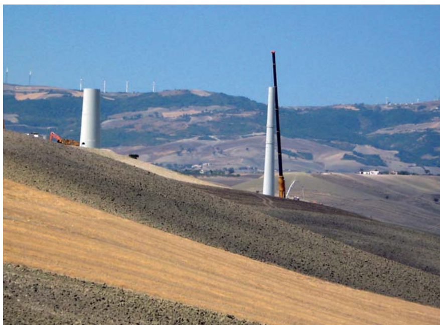
Construction of two concrete towers at ENERCON wind farm at Alberona (Province of Apulia).
