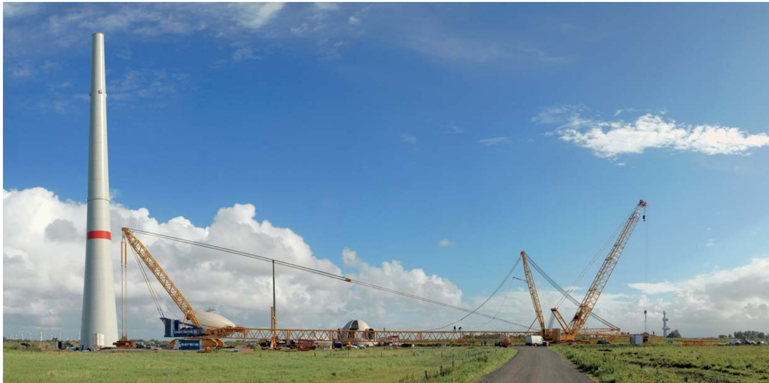
Crane lying on ground on Rysumer Nacken: In upright position, it measures a towering 180 meters and can lift up to 1200 tonnes.
