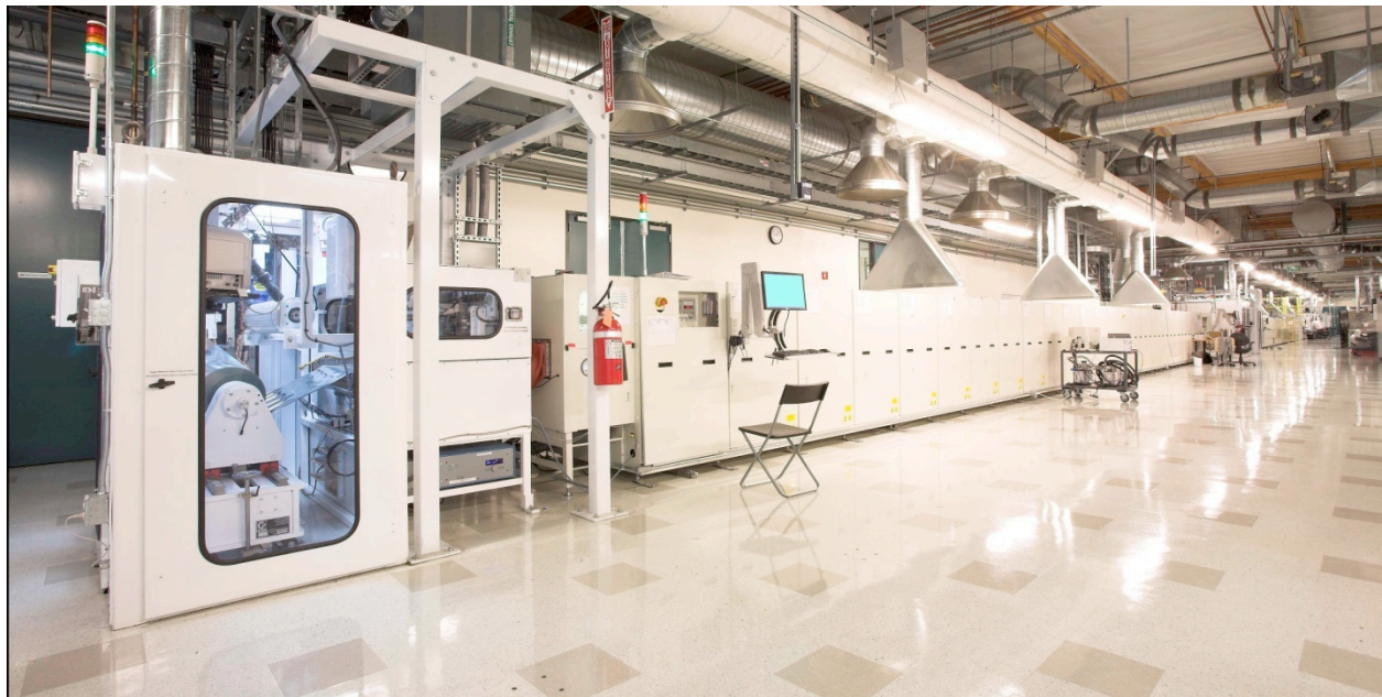
Figure 9: A Nanosolar roll-to-roll processing tool for rapid semiconductor formation, San Jose, California.
